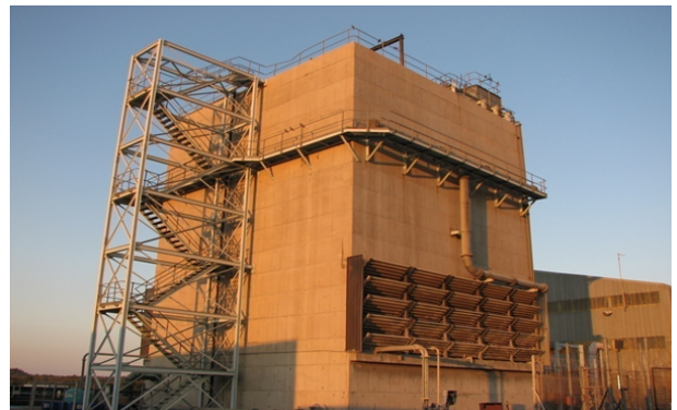
Siphumelele 1 Shaft Condenser Cooling Tower
