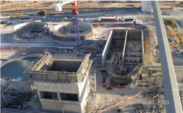
Amandelbult Surface Cooling Plant
