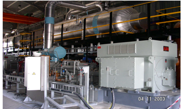
Amandelbult Ammonia Refrigeration Machine - 21mW(R)
